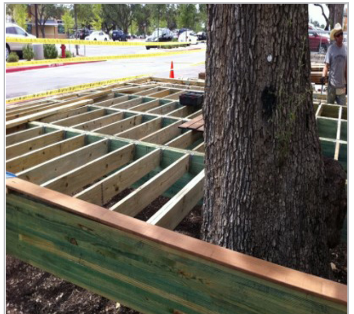
Power Preserved Glulam® Deck Application
