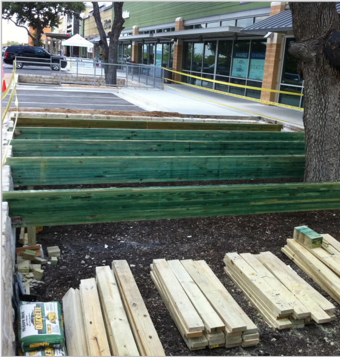
Power Preserved Glulam® Deck Application
